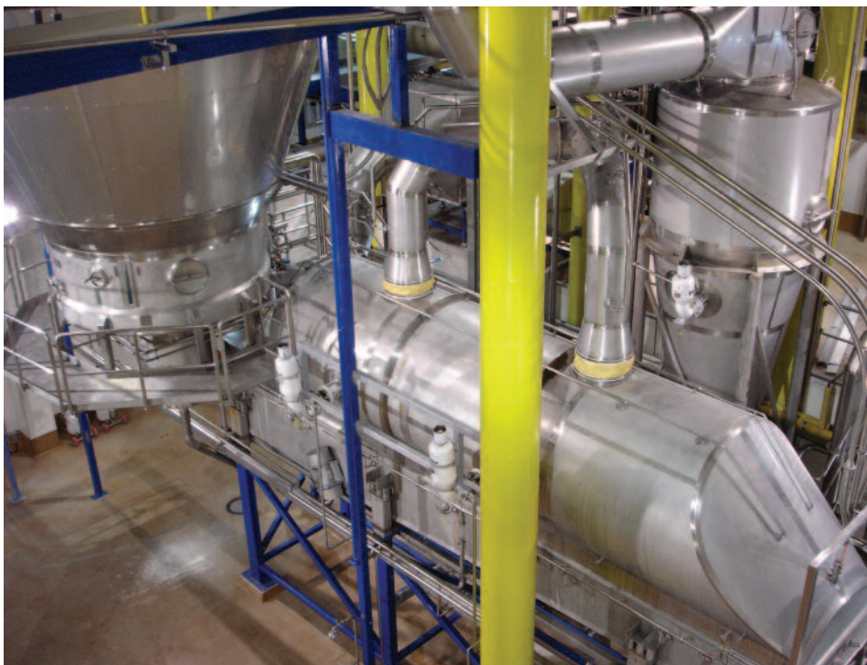
Spray dryer, its cone partially visible at left, has internal (foreground) and external (background) fluid beds for additional capacity, which improves the resulting powder's characteristics.
